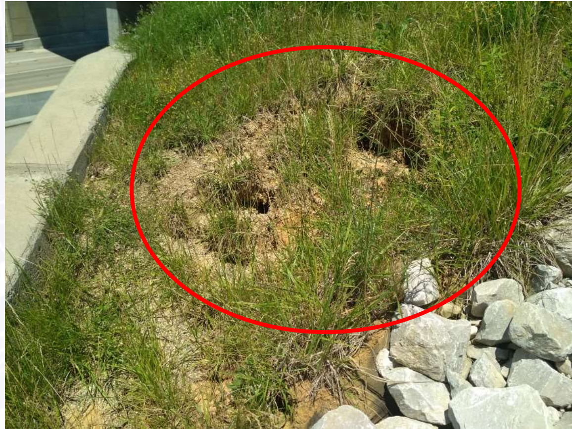
Subsidence due to loss of backfill
