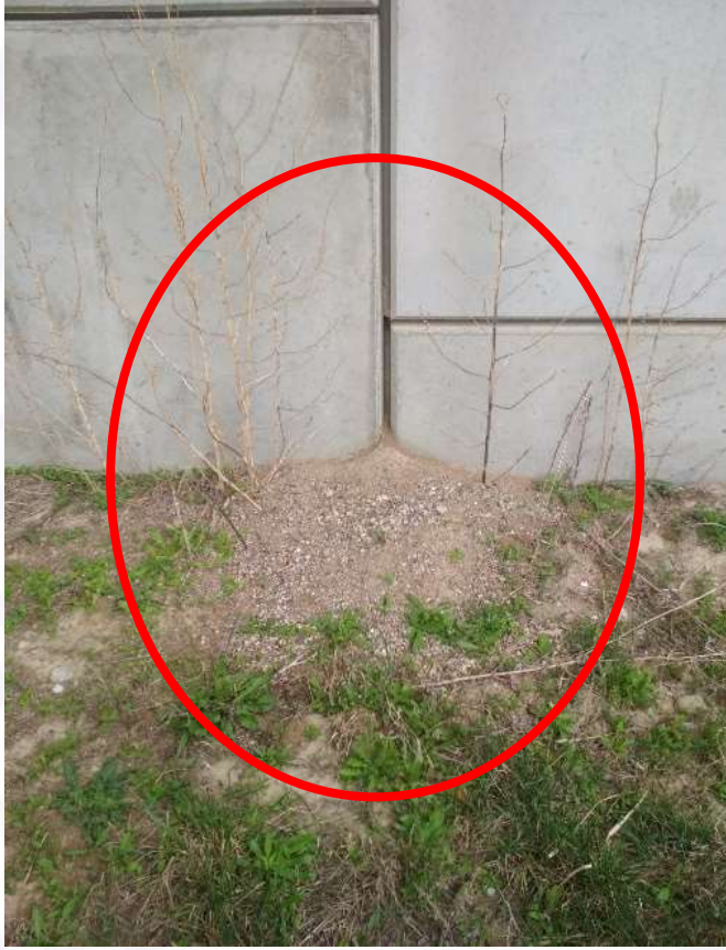
Loss of Backfill
